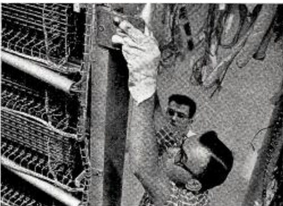
TELEPHONE SWITCHING FRAMES , like this one being installed in a Bell telephone central office by Western Electric personnel, are scheduled through manufacturing and shipping to arrive at central office locations — ready for installation — exactly on the dates they are required.
